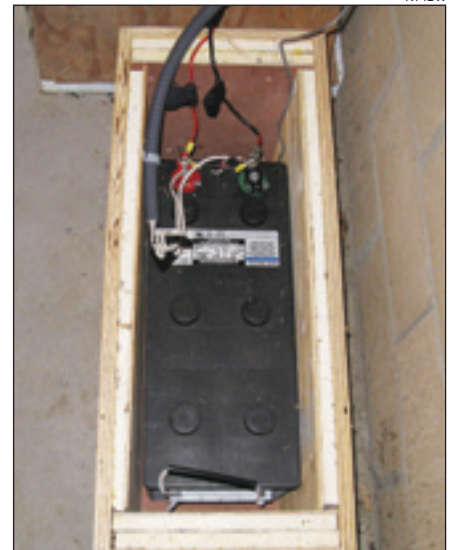
Figure 3 — Selected battery for our system, a Deka 12 V, 198 Ah unit. This battery weighs 130 pounds. Insulated battery box designed and constructed by Joe Koester, W4NSA.
