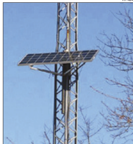
Figure 6 — 130 W PV panel on line in Tennessee.
