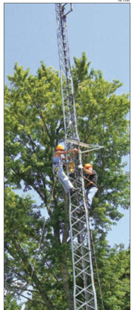
Figure 4 — Panel bracket installation by Al Perkins, KA1KIX, on left, assisted by KT4BW.
