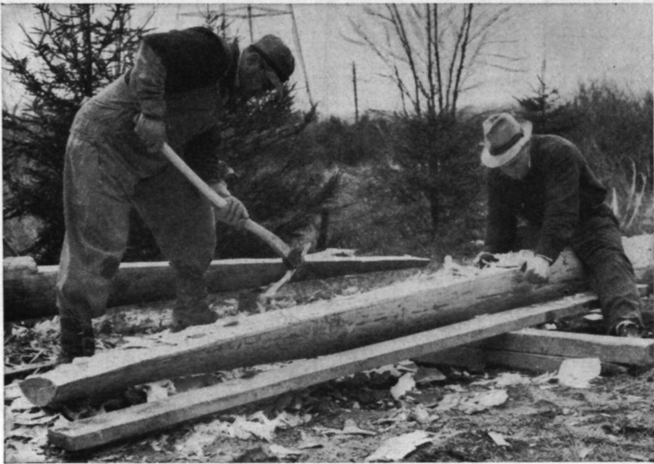
FIG. 3.113. Preparing the construction of a lap splice for large poles. (Photograph courtesy of National Broadcasting Company.)
