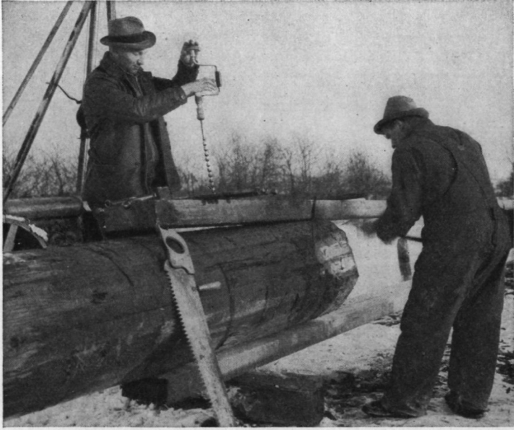
FIG. 3.112. The beginning of a pole-splicing operation and the construction of a butt-spliced pole. (Photograph courtesy of National Broadcasting Company.)
