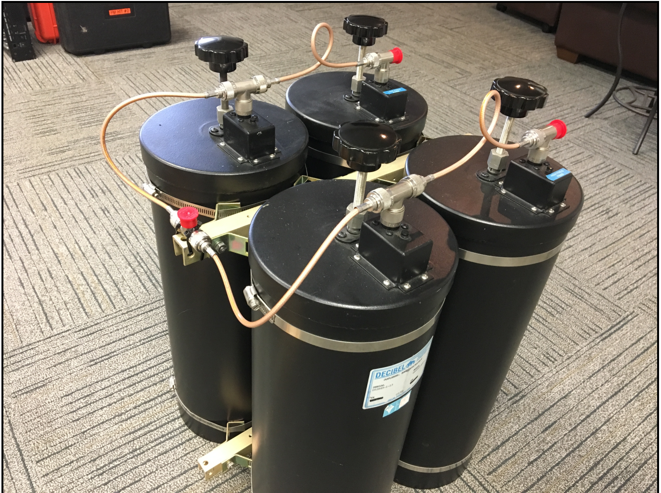
ASSEMBLED DUPLEXER AFTER CONVERSION
